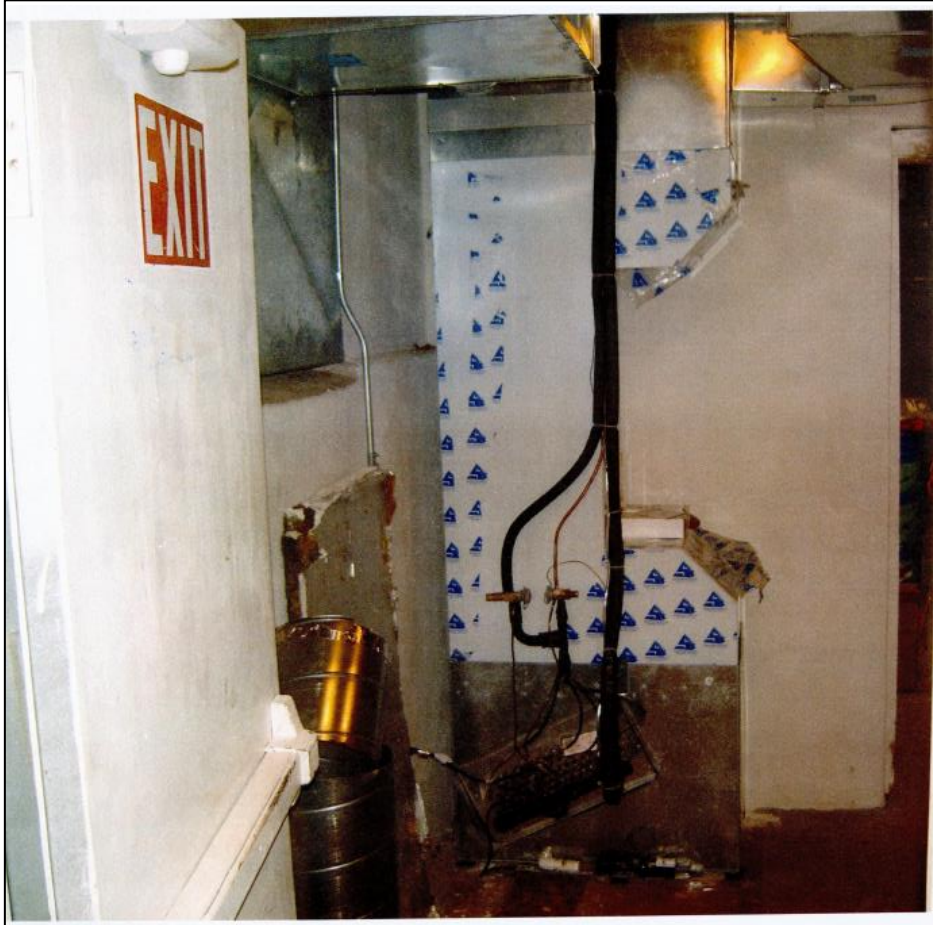
Figure 7 - A photo of a BPE ERV installed vertically in a latent only system
