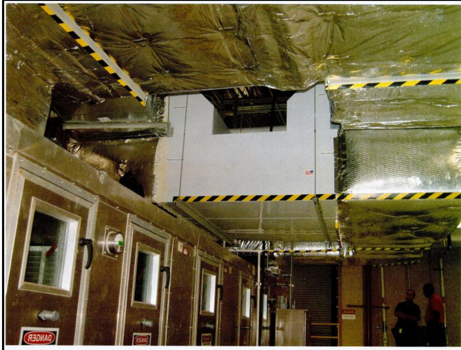
Figure 11 Image of a 6000 CFM BPE ERV hung from ceiling
