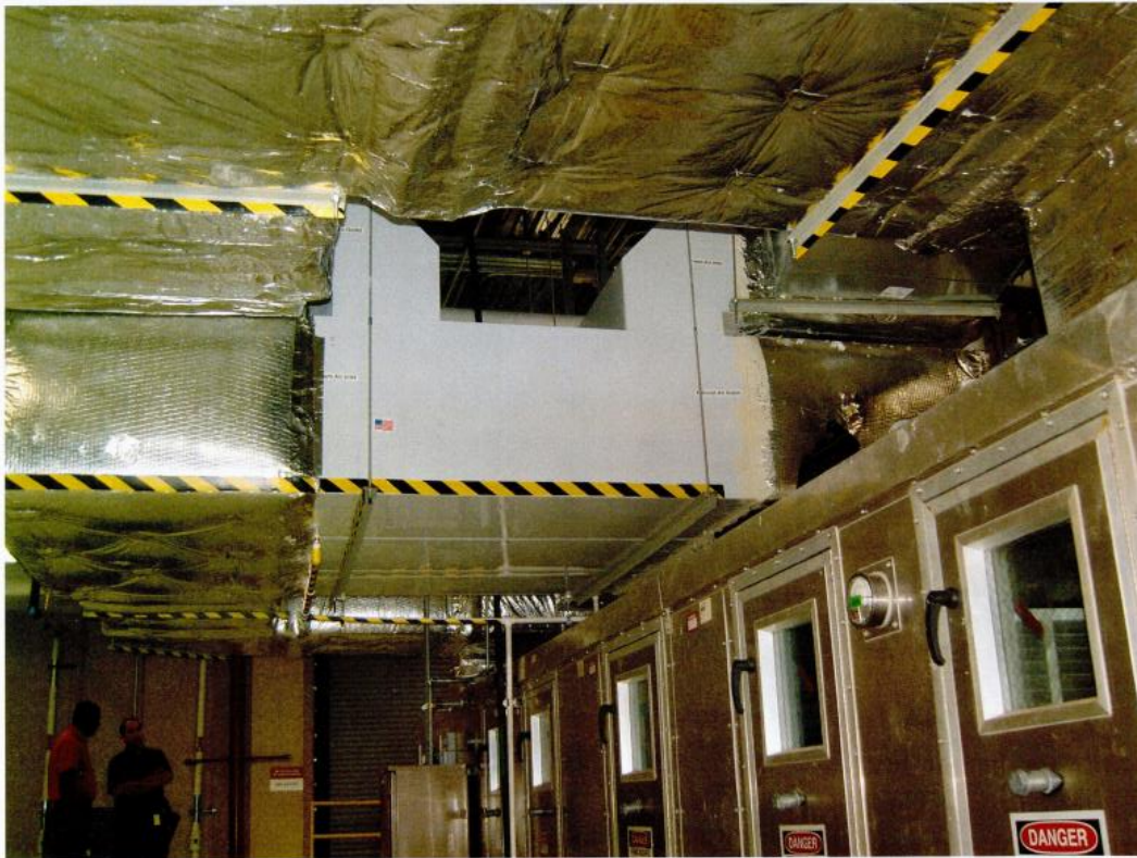
Figure 6 - a photograph of a 6000 CFM latent only system in an industrial facility
